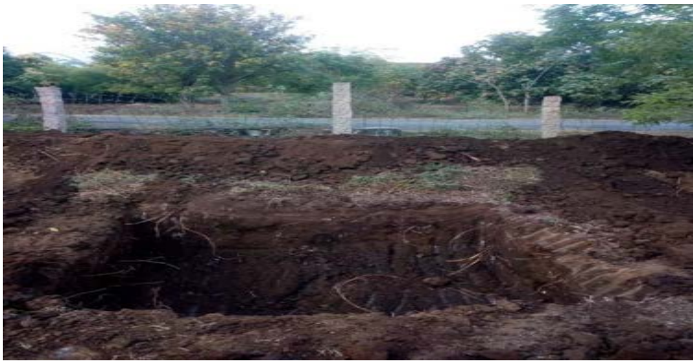
Catchpits constructed at Anjukulipatty watershed (S.No :999: Palanisamy )
